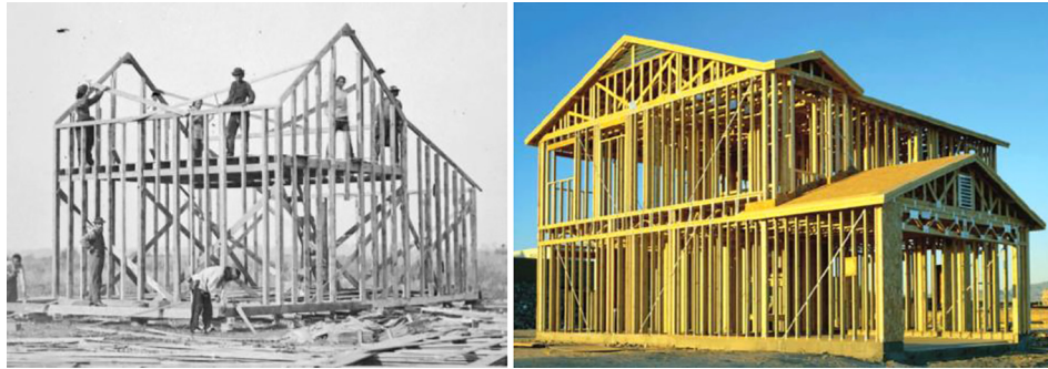
Fig. 15 Home construction in 1877 (left) versus current construction (right). Sources: National Endowment for the Humanities, 6 Architecture Curriculum at McGill University in Canada. 7
